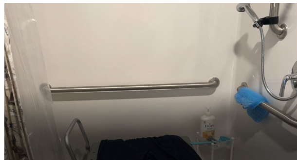
Resident accessible shower
