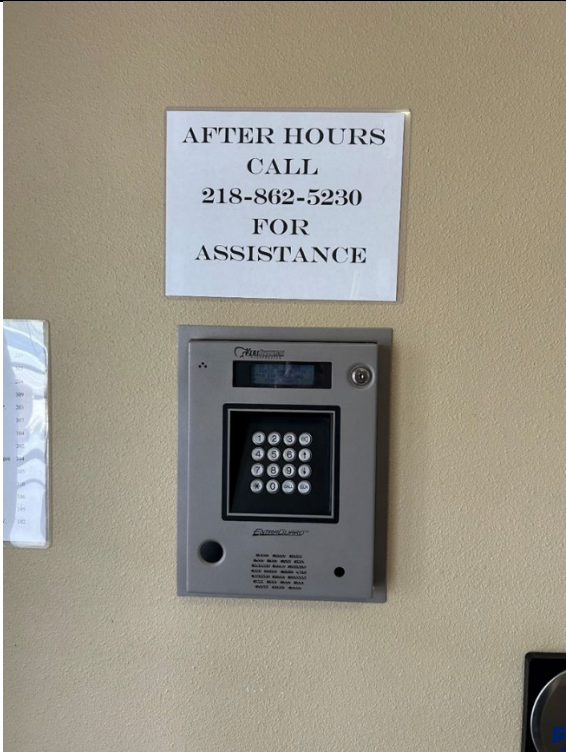
Call pad located at front entrance to the HCBS setting.
