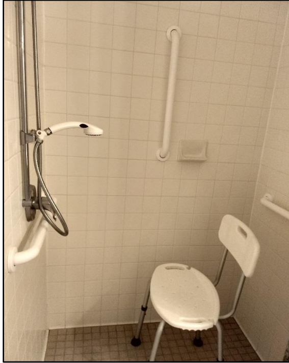
Accessibility accommodations in bathroom of living unit
